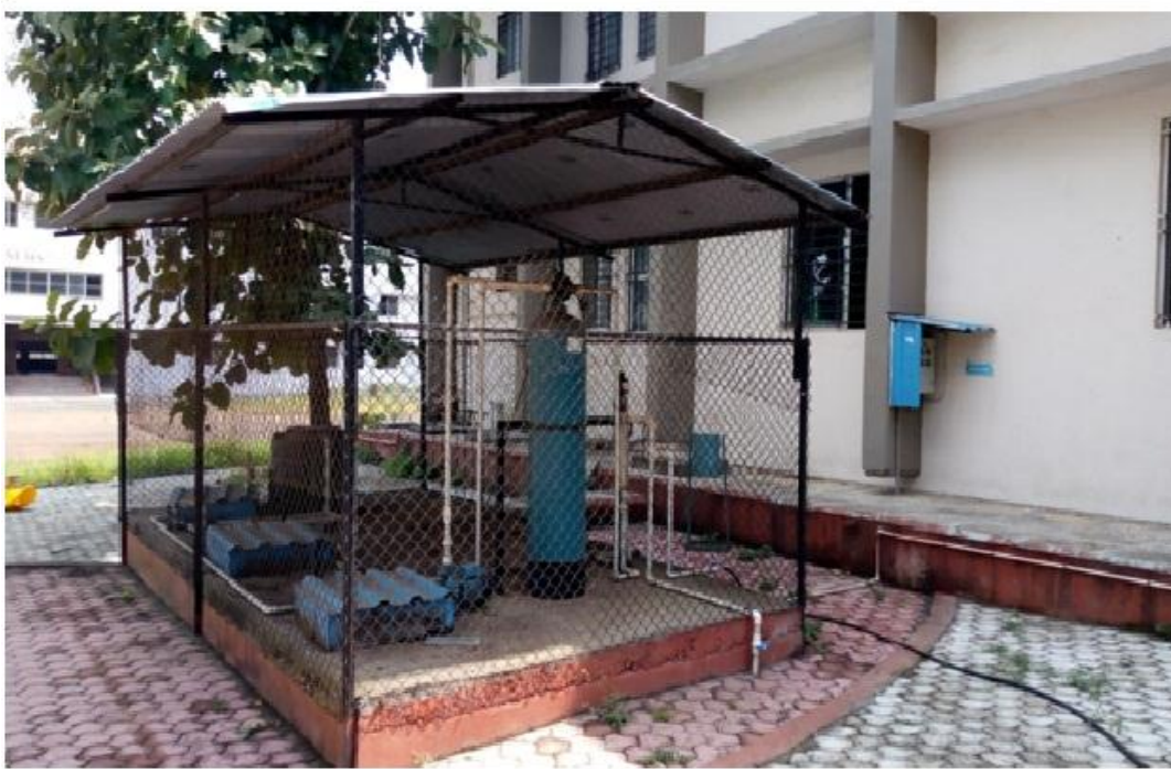
Plate No.3: STP near Library (10 MLD)
